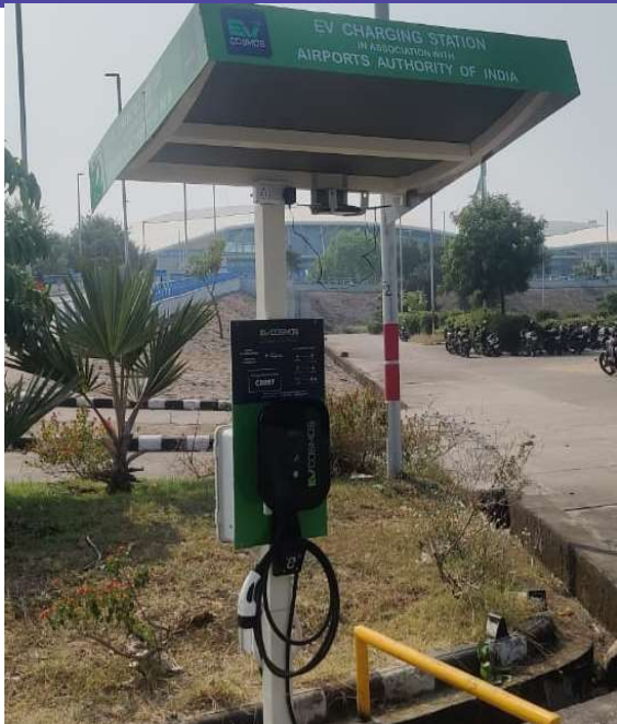
Public Charging – Bhopal Airport
